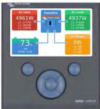
Color Control panel, showing a PV application
